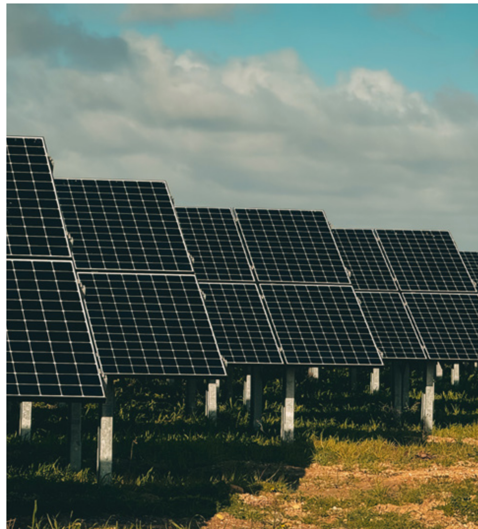
Above: The Solar Farm at the Fiumicino Airport, managed by Aeroporti di Roma Cover: Motorway section managed by Abertis in Brazil through Arteris
